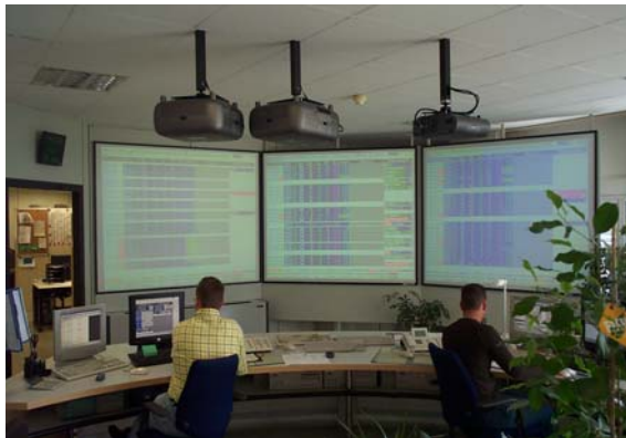
Fig. 1. Control room of DaimlerChrysler's automotive plant in Bremen, Germany
